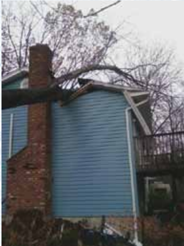
A fallen tree lies on a home in New Windsor, N.Y.
